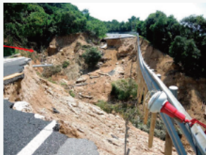
Collapse of a road embankment in the 2018 Japan floods (from Tsuchida and Hashimoto)
