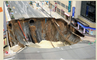
Collapse in Hakata (Nov. 2016 Asahi digital)
