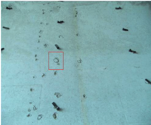
Damage of inside tunnel for verification (photo-shooting by digital camera)
